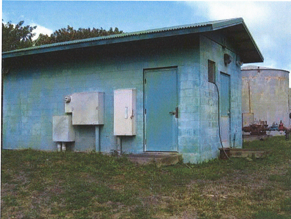
Photo No. 9: Hamakuapoko Well No. 2 Electrical Building (Makai North View)
