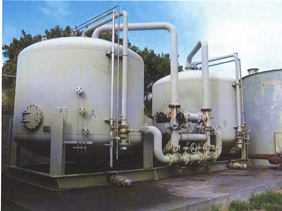
Photo No. 13: Hamakuapoko Well No. 2 Granulated Activated Carbon Units (East View)
