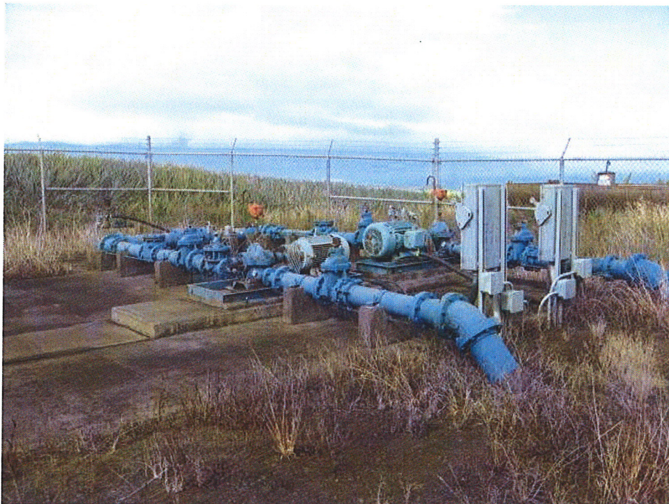
Photo No. 6: Hamakuapoko Well No. 1 Pumps (Northwest View)
