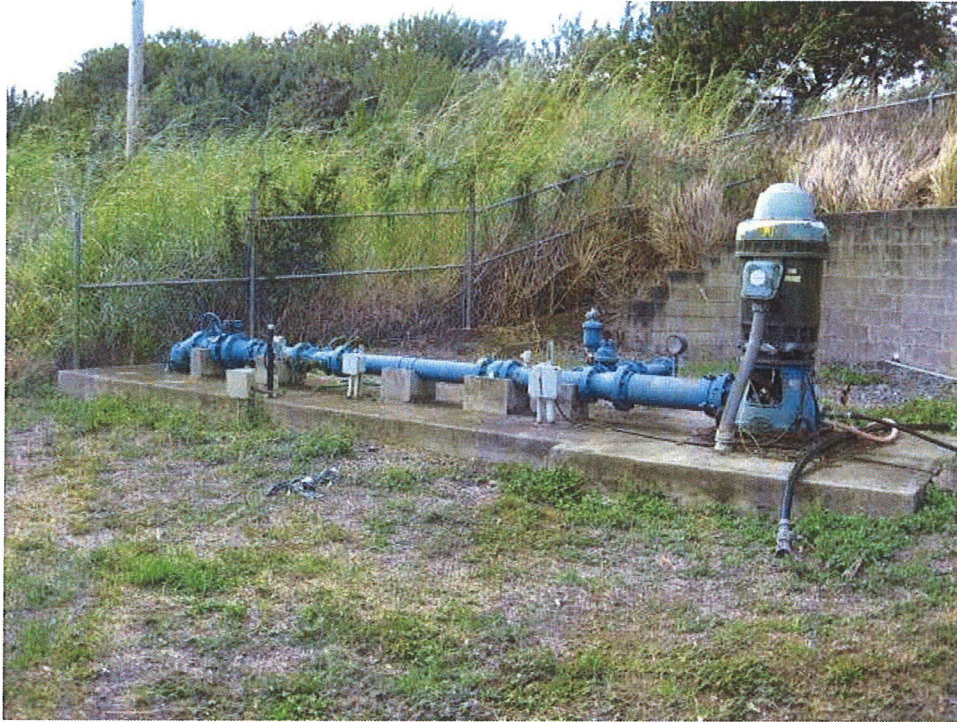
Photo No. 11: Hamakuapoko Well No. 2 Pump (South View)
