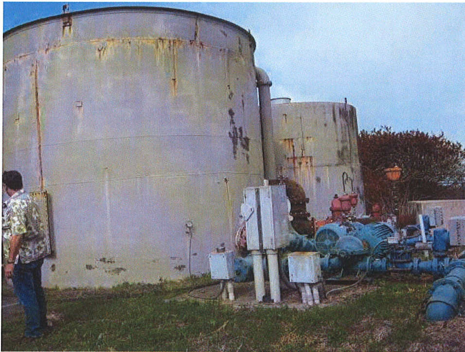
Photo No. 12: Hamakuapoko Well No. 2 Storage Tanks (Makai North View)
