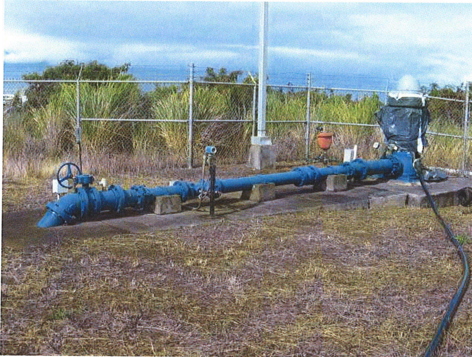
Photo No. 7: Hamakuapoko Well No. 1 Pump (West View)
