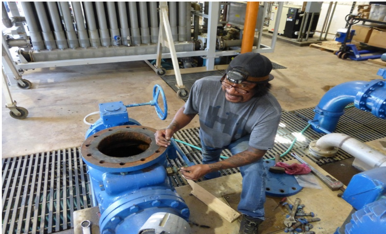
Water Treatment Plant Maintenance Mechanic | Federico Quitevis replacing the seal on a flange.
