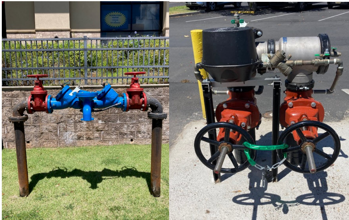
Photo Left: 4" Reduced Pressure Back-flow Preventer (RPBP) located at Maui Lani Parkway
