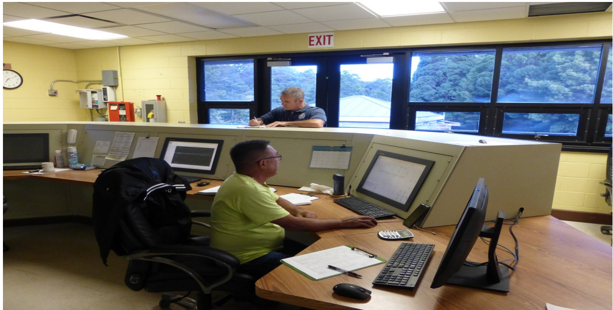
Piiholo Control Room with WTPO Grade IV operators Dale Kawahara (seated) and Phillip Noetzel
