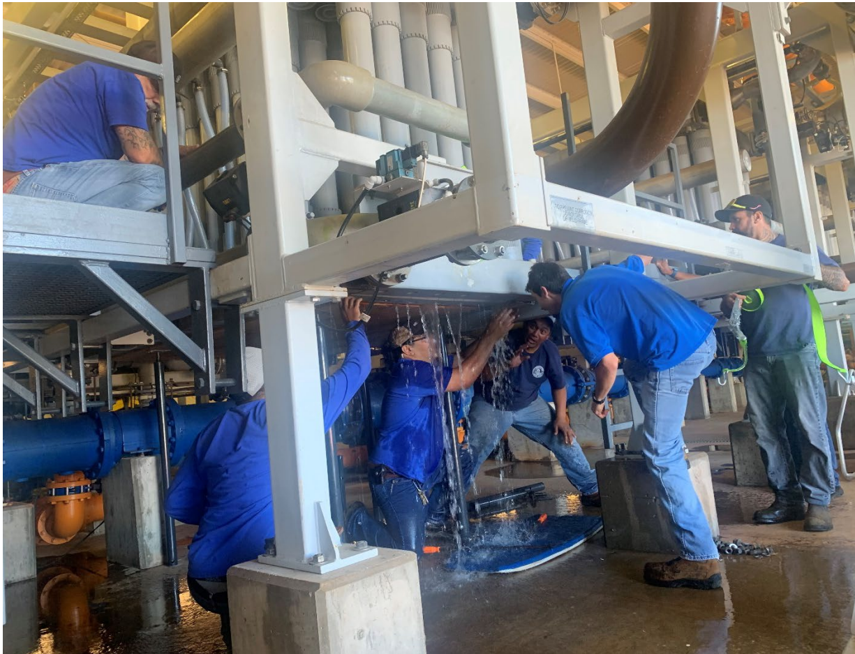
DWS Employees replacing a continuous microfiltration (CMF) unit block at the Kamole Water Treatment Facility.
