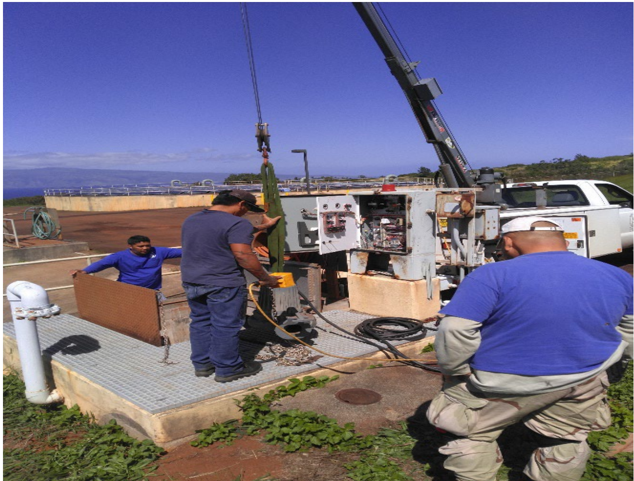
Pump and motor control replacement project at Mahinahina Water Treatment Facility from L-R: Brandon Wong WTPO IV; Frederico “Pocho” Quitevis, Water Plant Maintenance Mechanic I; and Chris Maeda, Plant Electrician/Electronics Repairer II.
