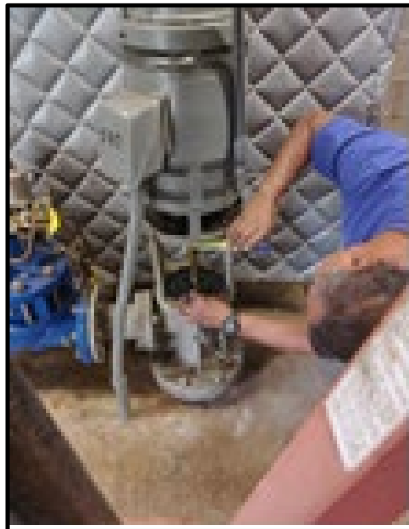
(Above:) Water Plant Maintenance Mechanic Mark Amano measures booster pump shaft for adjustments.
