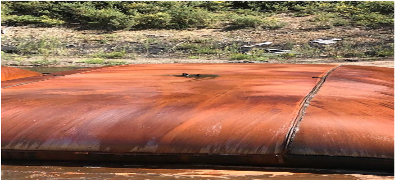
Permeable geotextile bag used to retain sediment during the cleaning of the 8.5 million-gallon pre-sedimentation basin in Olinda.
