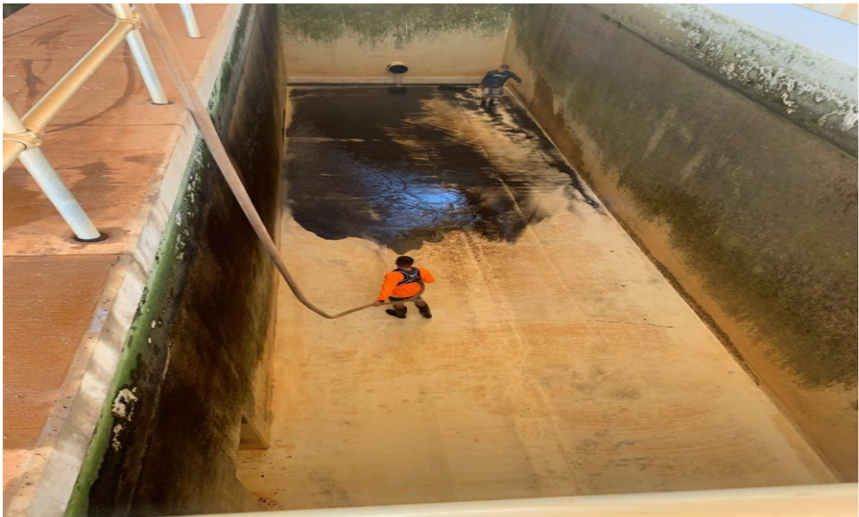
DWS Employees Water Treatment Plant Operator IV, Brandon Wong and Water Treatment Plant Trainee Ronald Kranchick Jr., cleaning the pre-sedimentation basin at the Lahaina Water Treatment Facility.
