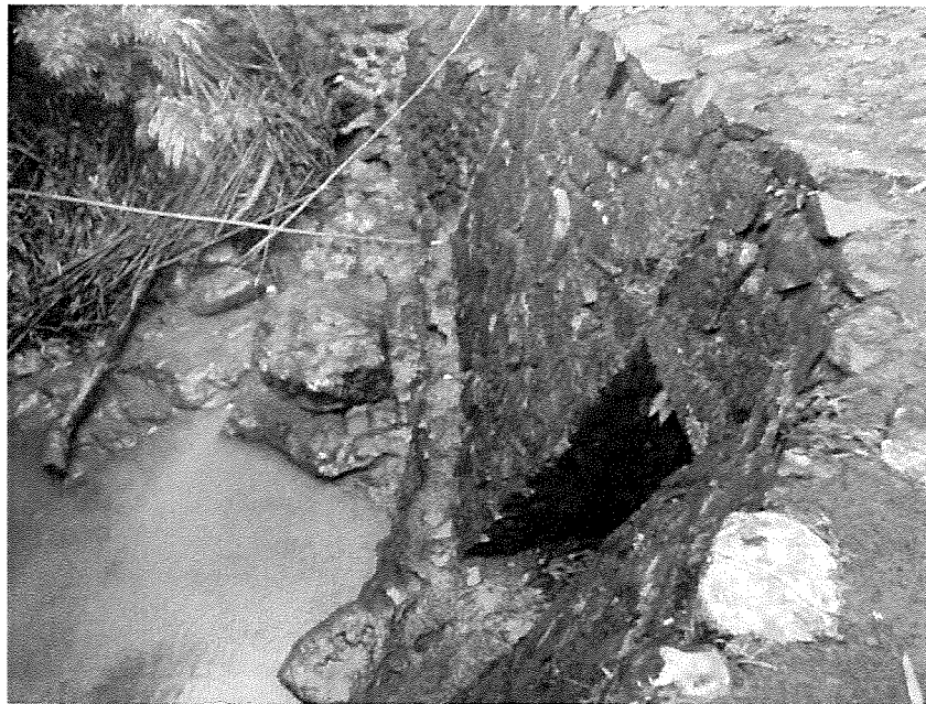
Figure 4-7. Photo shows below the diversion and is taken across the stream. Note there is only a trickle flowing from the gate. (3/12/2009; Tributary name: Kōlea (64003001); PBN: dk003p-017-031209; Surveyor: Kuamo‘o, D.; SBN: dk003n-031209; Lat. (DD): 20.87282, Long. (DD): -156.19005).
