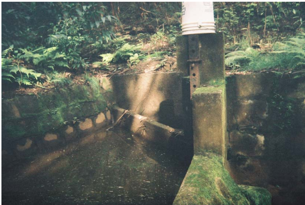
Better view of control gate.
