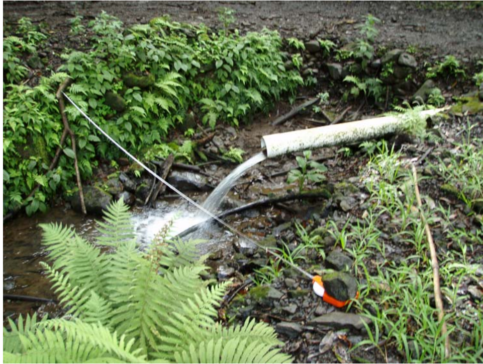
Pipe over Lowrie Irrigation ditch Hanehoi Stream (above Hana Highway and Ernie Schupp). Pipes make it difficult or impossible for upstream migration of native animals except at flood flows when the diversion is completely overtopped by the stream flow.
