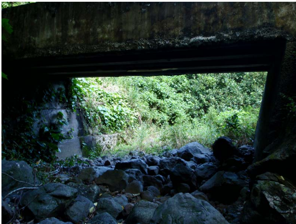
Figure 4-6. Photo shows a dry stream bed under Hāna Highway Bridge downstream from survey site 16. (12/9/2008; Tributary name: Punalau (64008001); PBN: sh016p-272-120908; Surveyor: Hau, S.; Habitat type: No Water; SBN: sh016r-120908; Lat. (DD): 20.86171, Long. (DD): -156.16972).
