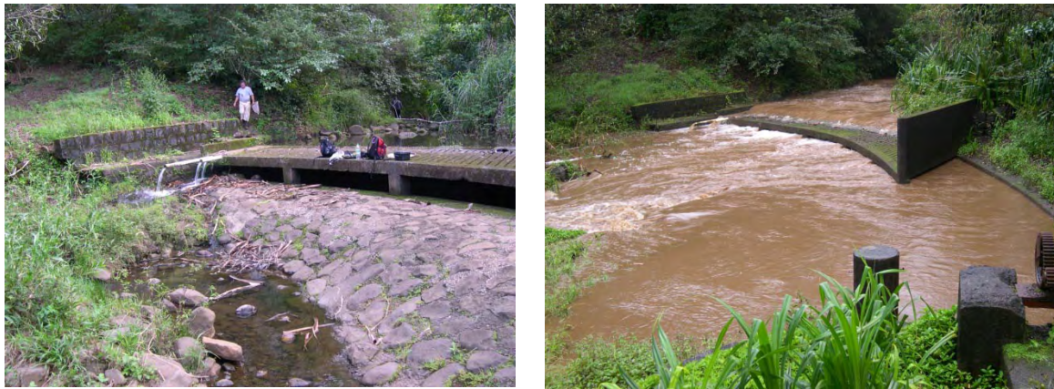
Figure 13. Two images of Honopou Stream, Maui at low (left) and high (right) flows. At low flow the barrier is a complete blockage to upstream migration and at high flow most of the water flows through the diversion structure. As postlarvae move upstream through the structure, many would be entrained in the diverted waters and removed from the stream.
