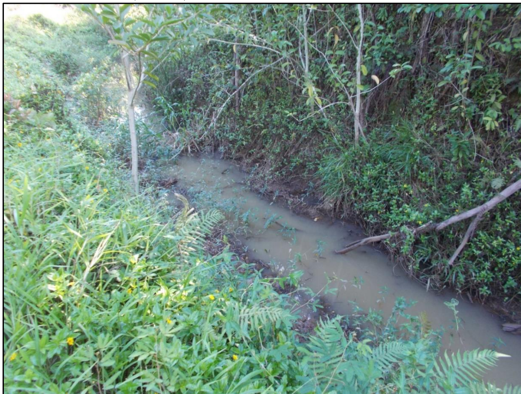
Figure 13. Lowrie Ditch, a typical section of the ditch along the east side of the Kapala'alaea Reservoir. View facing north. MASON, 2023.
