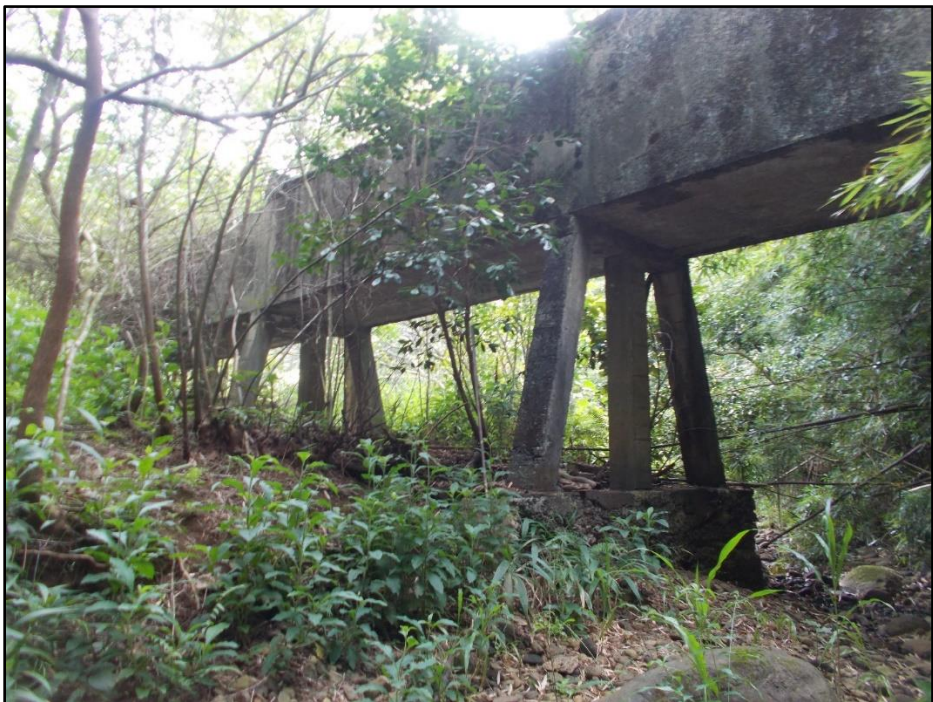
Figure 23. Concrete flume carrying Lowrie Ditch over the Piiloi Stream bed. View facing southeast. MASON, 2023.
