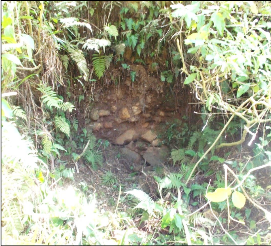
Figure 12. Outlet portal of the reservoir on the downstream slope of the dam. MASON, 2023.
