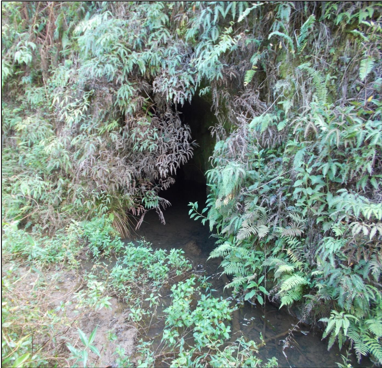
Figure 21. Kapala'alaea Intake to the Lowrie Ditch from Piiloi Stream. Note this intake provides water to create a downstream current in the ditch. View facing southeast. MASON, 2023.
