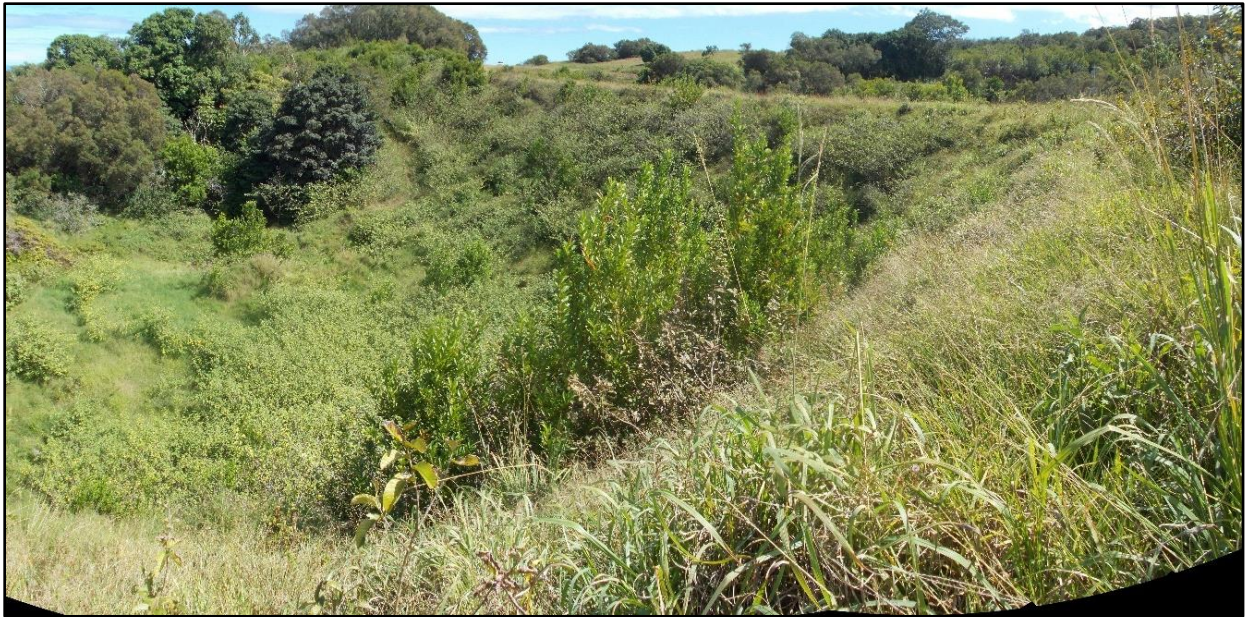
Figure 10. The downstream slope of the dam. Note the dam crest in the right background. View facing northeast. MASON, 2023.
