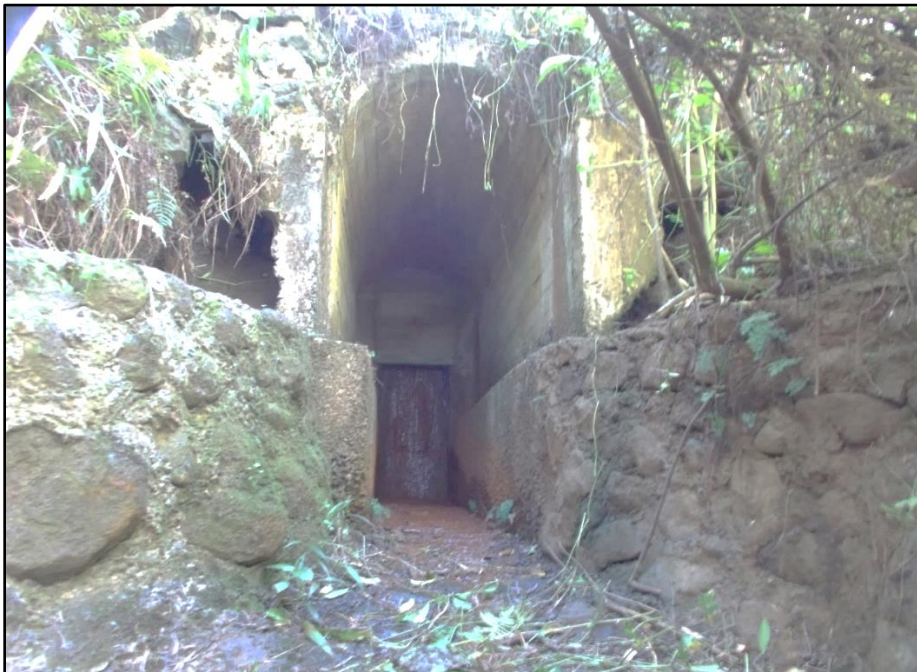
Figure 20. Arched concrete outlet portal of the ratchet gate. Note the steel gate panel in the rear that is closed against the rectangular opening to the ditch. View facing east. MASON, 2023.
